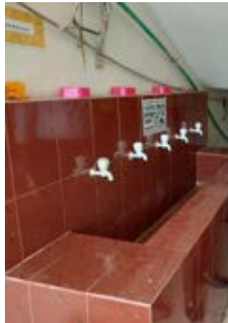
Fig. 9 water collection basin of 5 outlet
